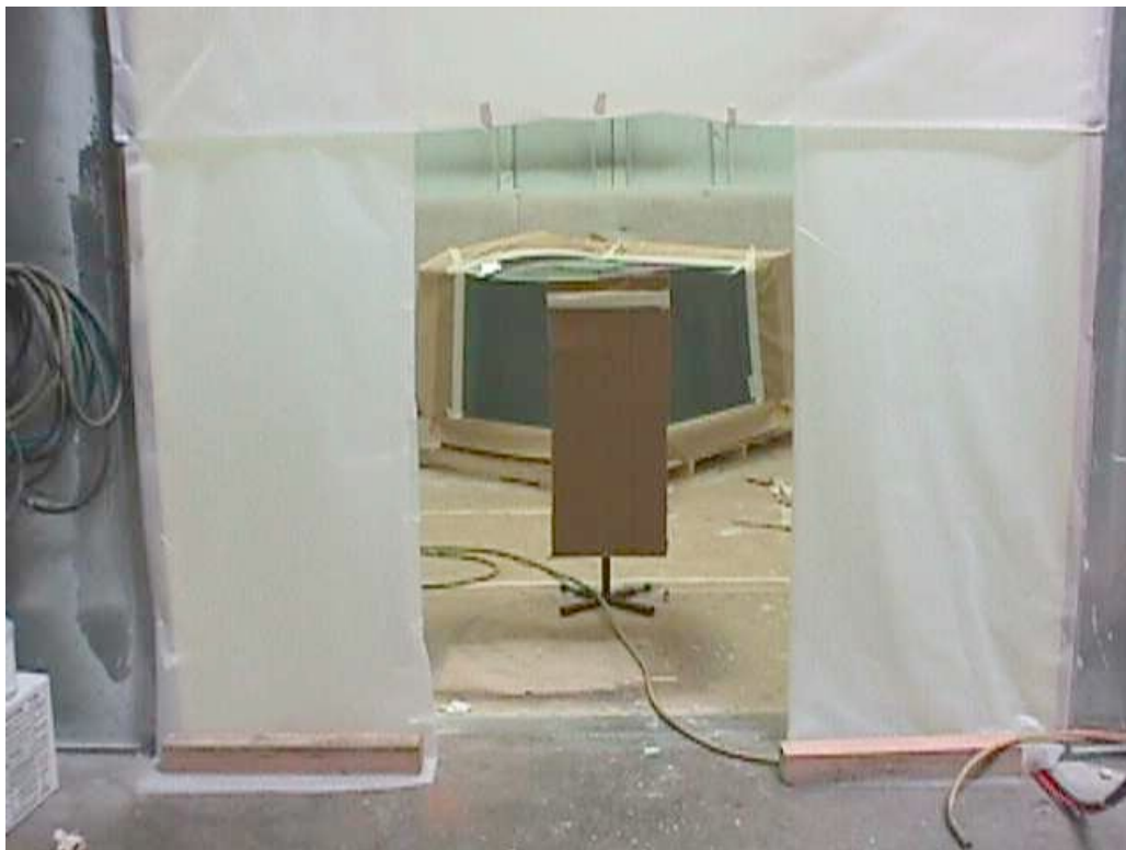
Figure 1 – Photographs of Spray Booth as a Temporary Total Enclosure
