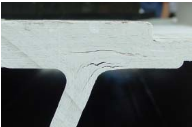
Figure – 2 Fiber delamination at joints of unidirectionally pultruded panels.
