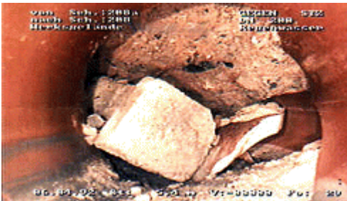
Figure – 3. Breakage and Collapse of a Concrete Pipe
