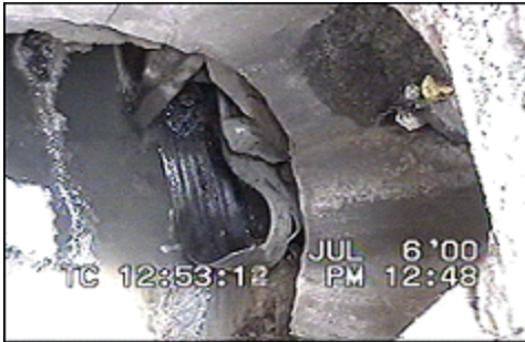
Figure – 2. Subsidence of a Concrete Pipe
