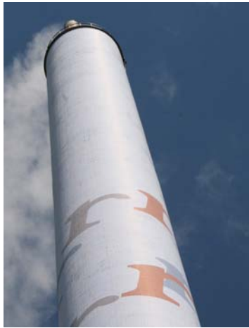
Figure 1: CFRP strengthening of a chimney in Sweden. The chimney was painted after strengthening
